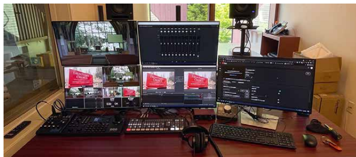
Fauntleroy tech room.
